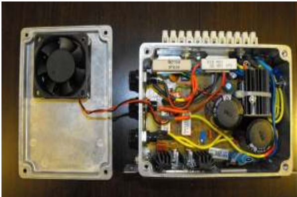
Photo 8: Switching Charger used in the project
