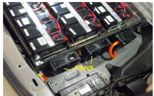
Photo 6: Cooling and ventilation fans
