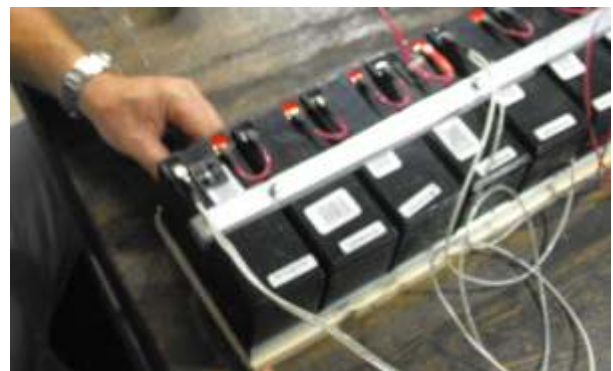
Photo 5: Installing the 12 Volts 7.2 Amp/Hour batteries in Series.
