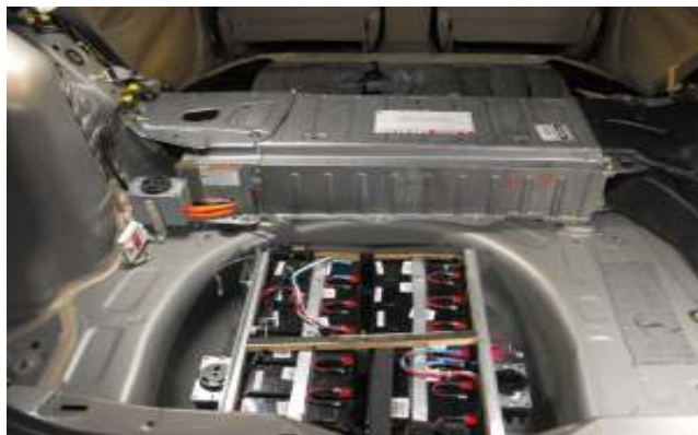
Photo 2: Lower battery pack
