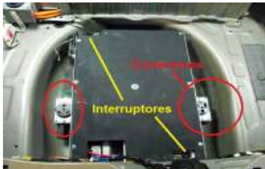
Photo 1: Lower Battery Pack - Switches
